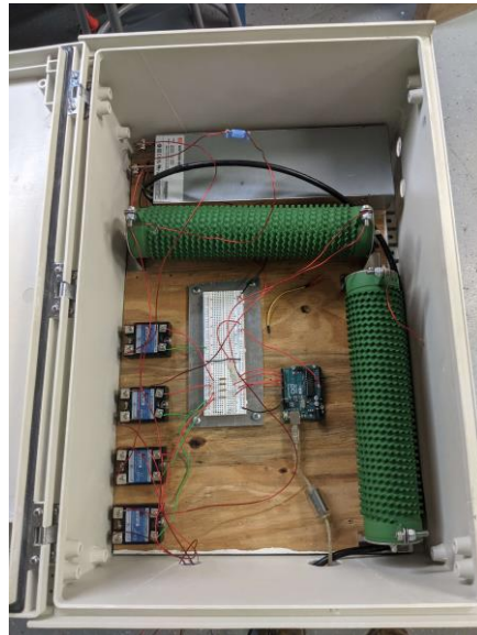
Figure 22: Setup of Electrical Components
